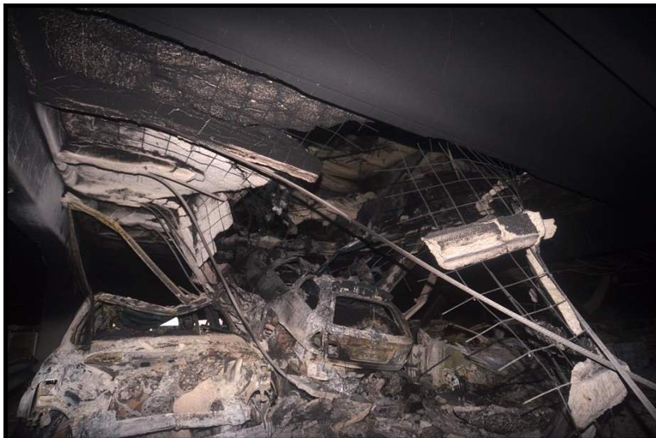
Failure of concrete as a result of the fire
