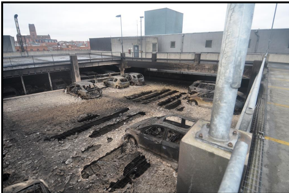
Fire damage on ramp leading to level 7
