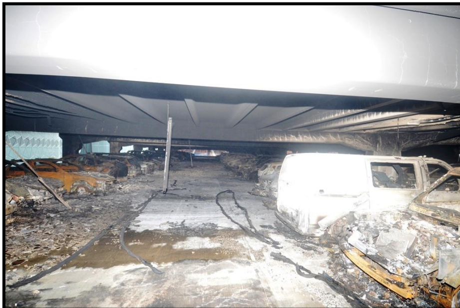
Fire damaged vehicles on level 3 in area where fire started
