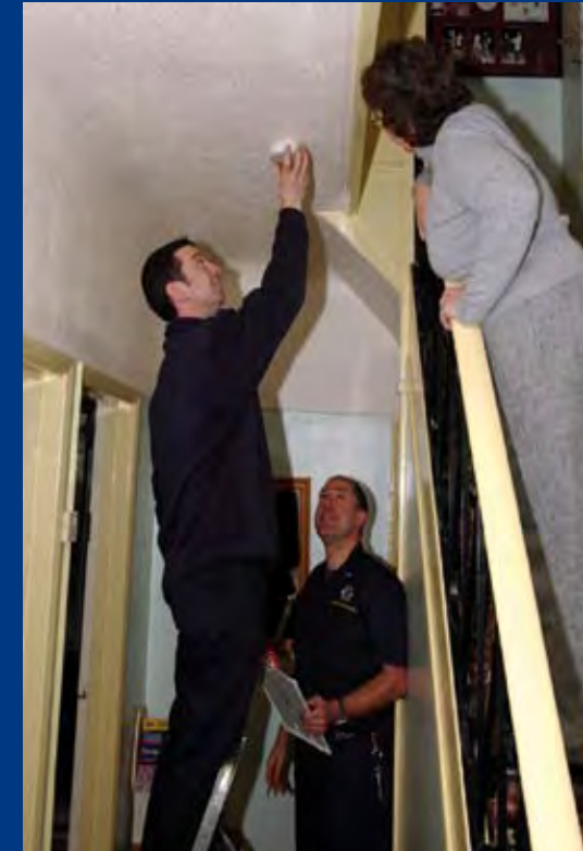
FREE smoke alarms being fitted by two firefighters whilst carrying out a Home Fire Safety Check.
