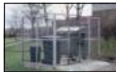
Correctly sited & secured bins
